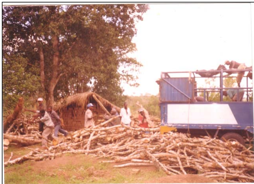
Photo 6: Kwafungo MSE operators loading materials for constructing a building to be used for training purposes.
